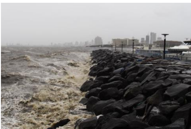
Figure 11. A breakwater in Manila Bay during the time TY Mangkhut passed through Manila (15 September 2018)
