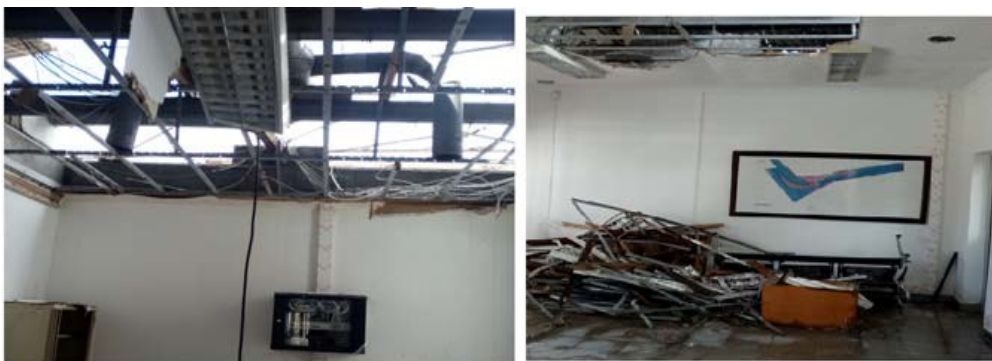
Figures 6: Illustration of the INAHINA's Office upon the occurrence of cyclone Idai. From the figure it is possible to see the damages on the computer equipment, ceil, and furniture.
