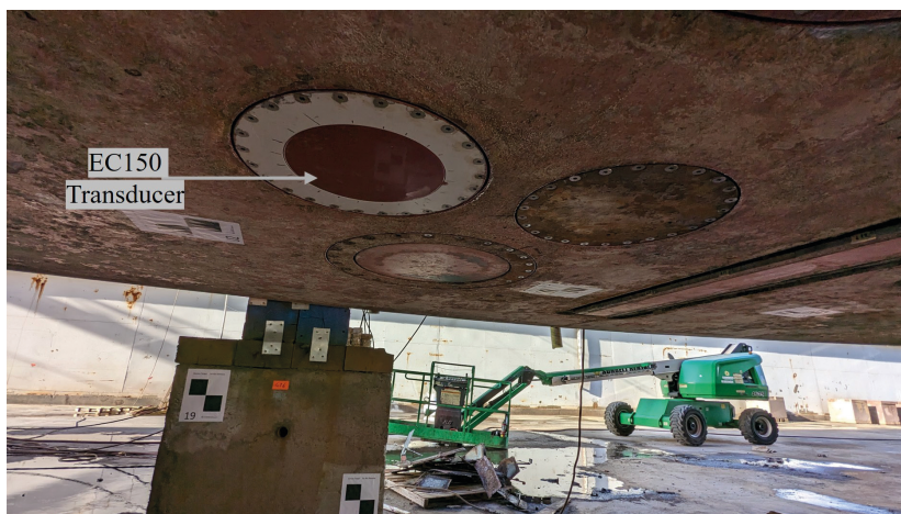
Fig. 8 Newly installed EC150 transducer.
